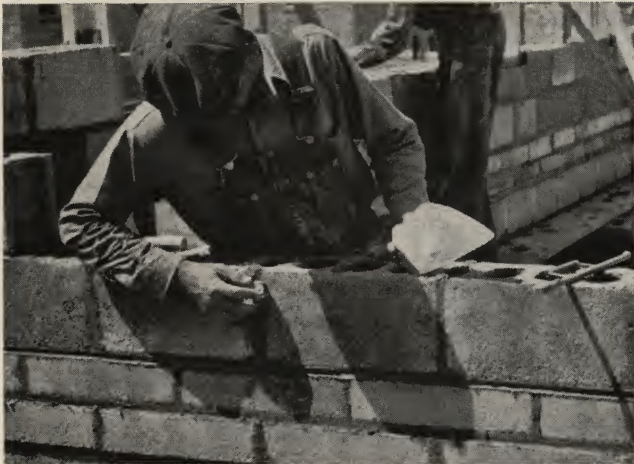
1—Mason rubs the vertical joint with a flat fragment of concrete unit to compact the mortar and obscure the joint.
